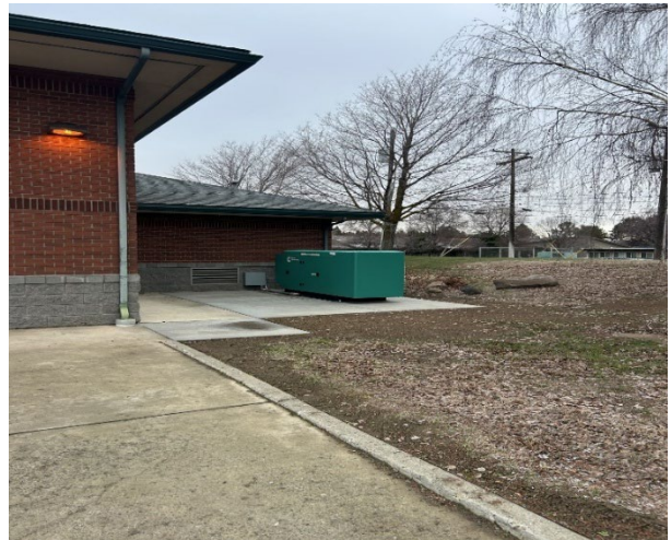
New emergency generator at Station 93
